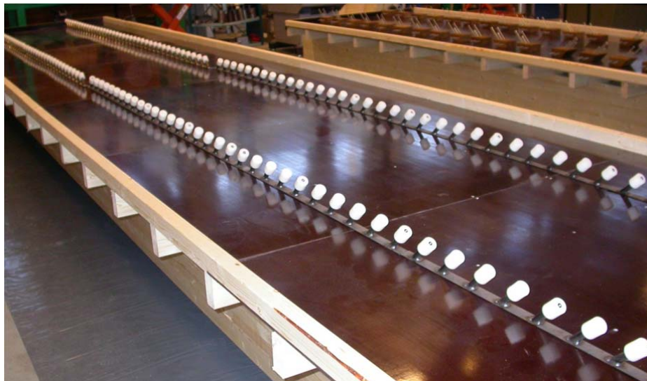
Figure 122: formwork before the casting of the concrete, with the connection system T12
