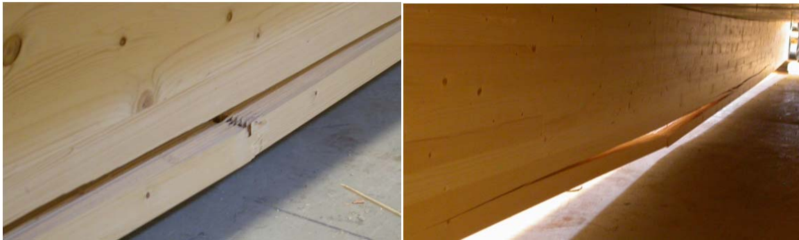
Figure 126: first failure of the system, due to the breaking of one finger joint in one timber beam
