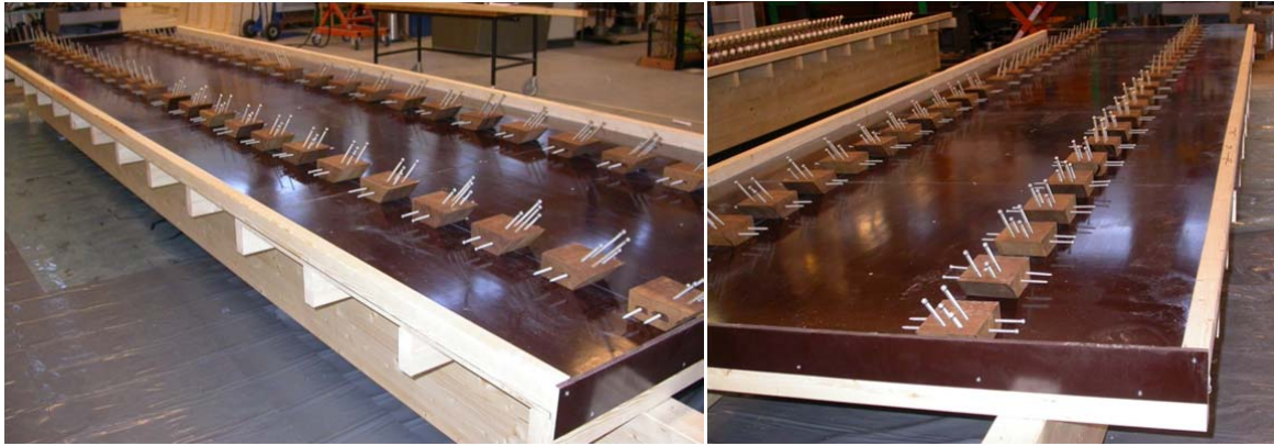
Figure 106: formwork before the casting of the concrete, with the connection system F45
