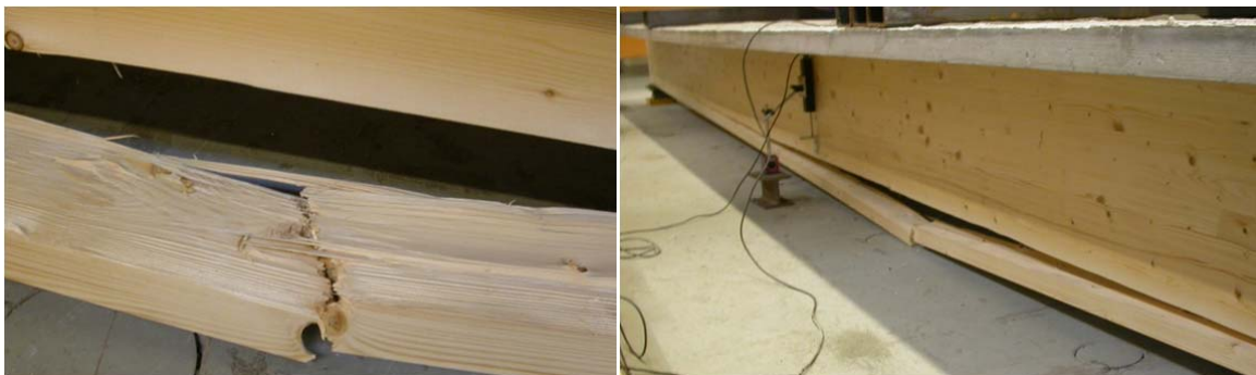
Figure 127: second and final failure of the system, due to the breaking of one knot in the other timber beam
