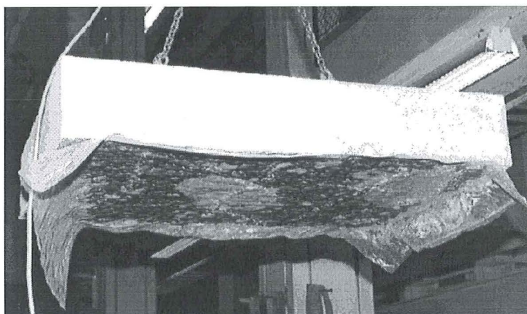
Figure (4.17) Bottom surface of the slab after performed test on ground covered by plastic sheeting.
