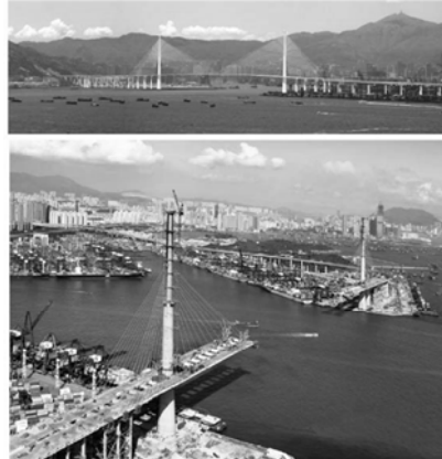
Figure 4-30: The Stonecutters Bridge (currently the largest cable-stayed bridge in the world) under construction.
