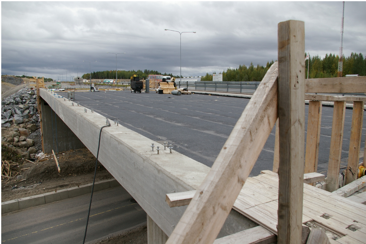
Figure A - 4: The bridge deck of Särkijärvi Bridge when it was being constructed (photo by K. Nikula).
