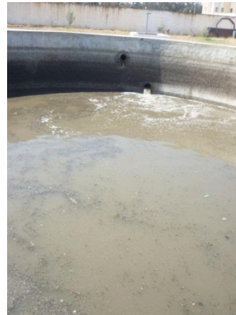
Figure 4.13. The water at the pumping station PS1 is not of good quality due to the large amounts of wastewater being received to SE3.
