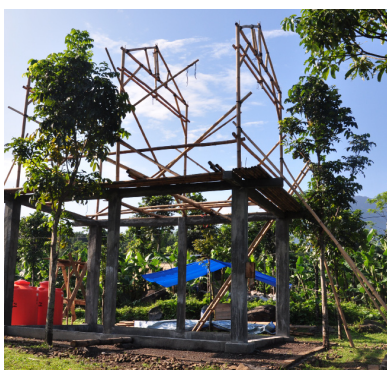
Treatment station, Lalandon.
