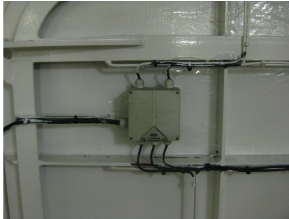
Figure 5: Plug in cubicle on board a cruise ship (Costa Luminosa)
