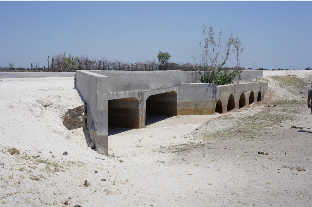
Figure 12. This bridge did not hold last big flood in 2010.
