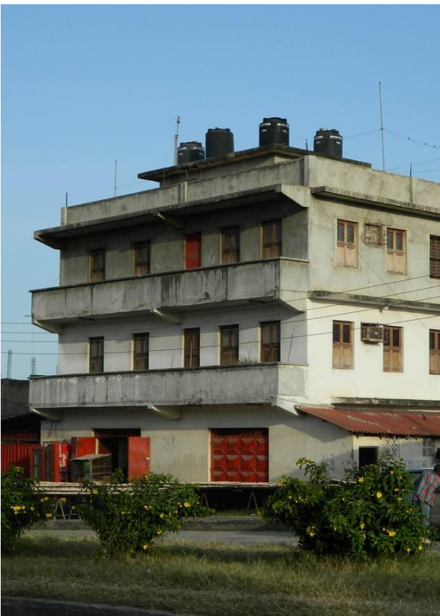
Fig 4.14 Water tanks placed on the roof to get pressure
