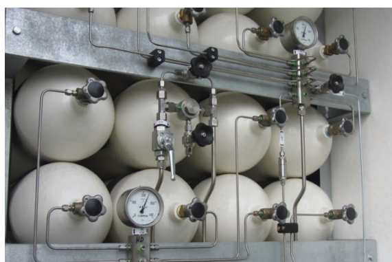
Figure 7 Upgraded biogas stored in tanks
