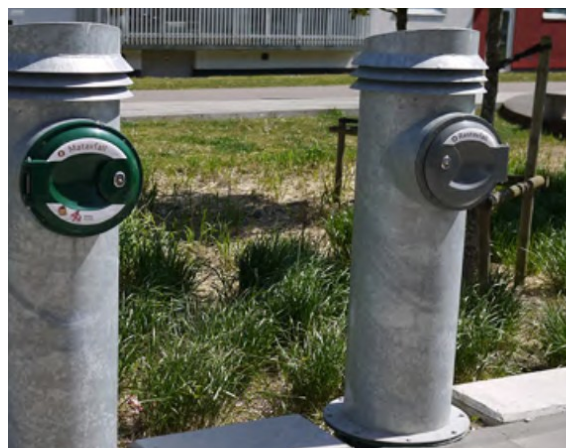
Figure 8. Waste station feeding underground waste infrastructure. (Source: Malmö stad, Western Harbour Guide)
