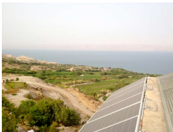
Figure 4, Solar PV installation Sehatty resort. Dead Sea, Jordan. Photo: Emma Åberg, IIIIEE.
