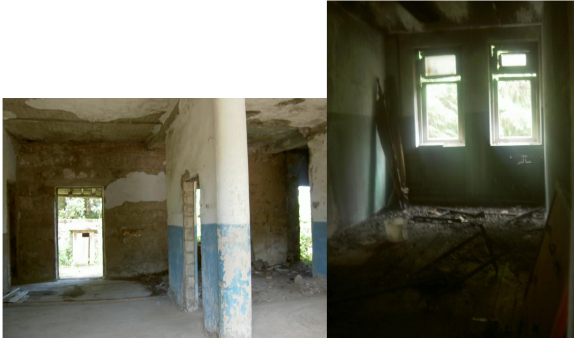
Figure 4. Photo on the left shows a non-renovated part of the building in which the health center of Akhlo was located. The clinic was situated on the second floor. Photo on the right depicts a part of the health center in Shori that was damaged in the fire. The women's groups as critical issues chose renovation of the two health centers.
