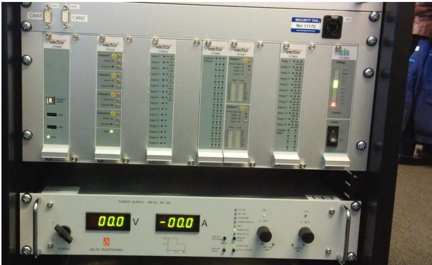
Figure 2.2 The VT-system with its modules mounted in a 19" rack cabinet. Real-time module to the far left. Power supply below the VT-system.
