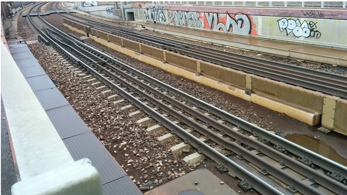
Figure 17. The transition zone on the north side of the bridge, illustrating the design with the associated guard rails, dilatation device, ballast box and direct rail fastening system.
