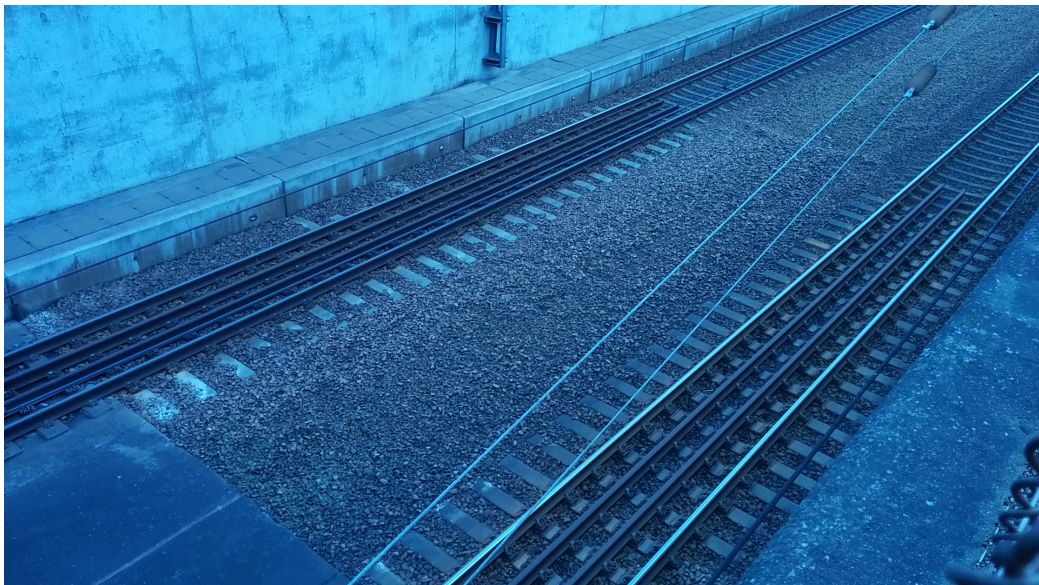
Figure 7. The transition zone at the entrance to Drogdentunneln, with auxiliary rails and longer sleepers.
