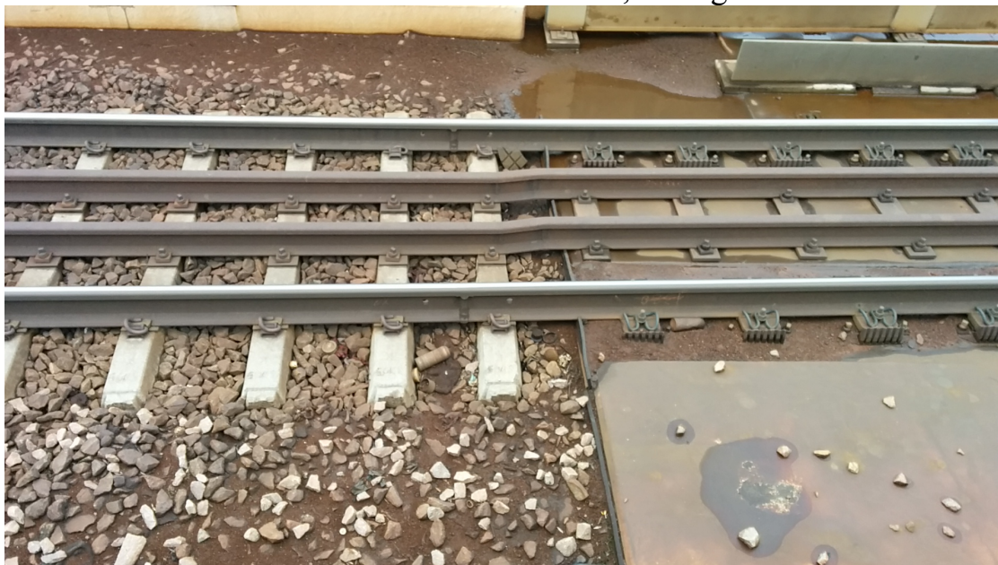
Figure 18. Transition zone on the north side of the bridge, illustrating the existence of fines and water collection in the ballast box.
