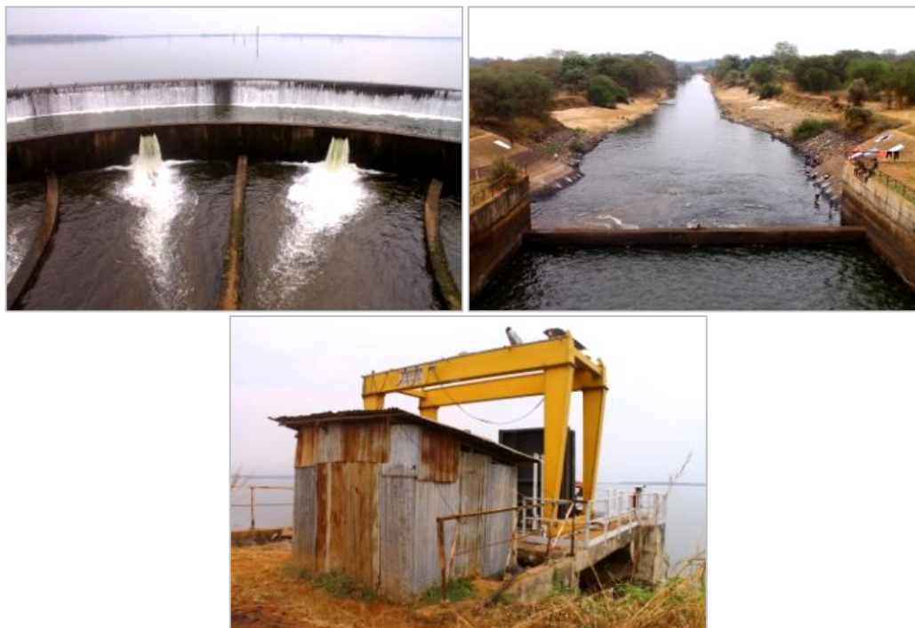
Photo 2-4: The Alwero dam and its spillway, The Alwero river downstream from the dam Intake of the Alwero dam that allows water flow to the main canal Source: the Author
