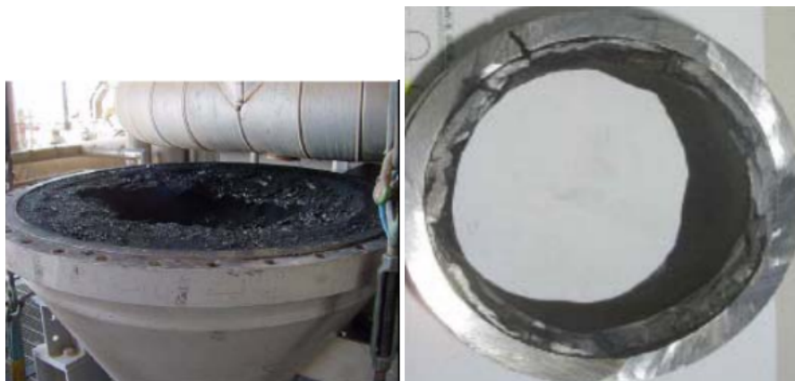
Figure 7.7 Coke accumulation in pipes.
