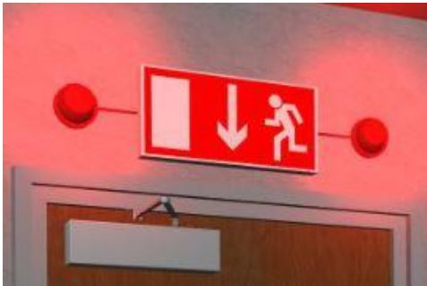
Figure 11. Sign 11: red background, running man pictogram, red flashing lights.
