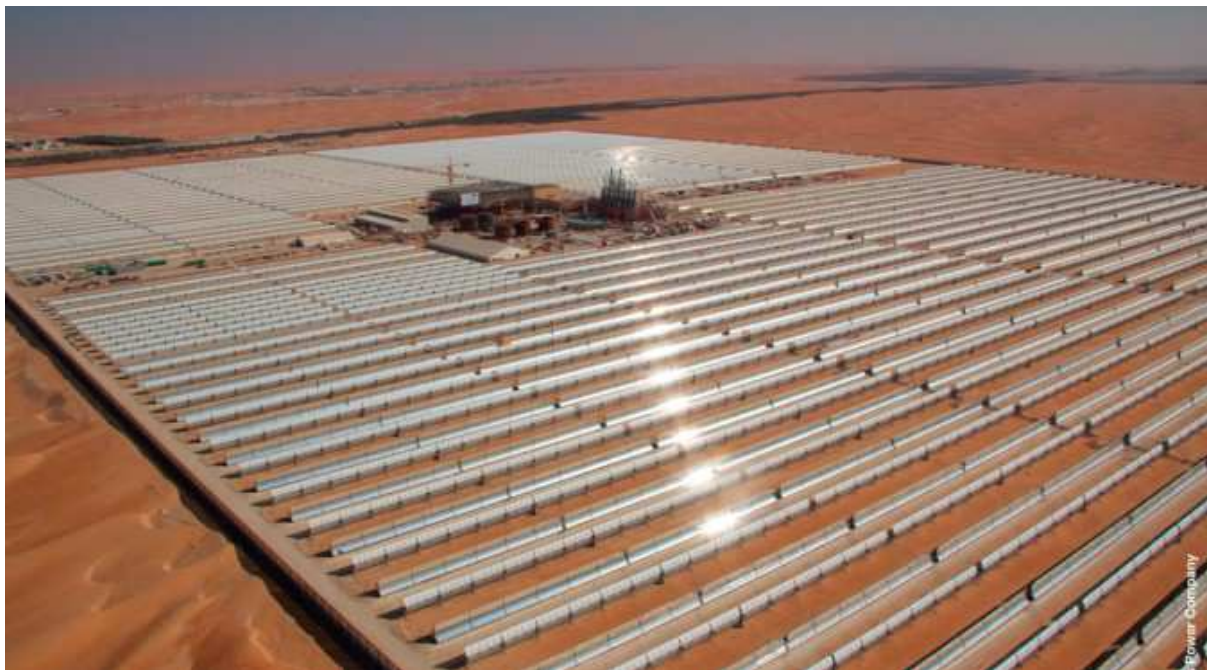
Figure 6: Construction site of NOOR 1 in Ouarzazate. Source: http://www.evwind.es/2014/10/20/first-concentrated-solar-power-csp-plant-in-morocco-solar-energy-project-to-open-in-2015/48190 The power of the sun: CDA of the Moroccan solar sector
