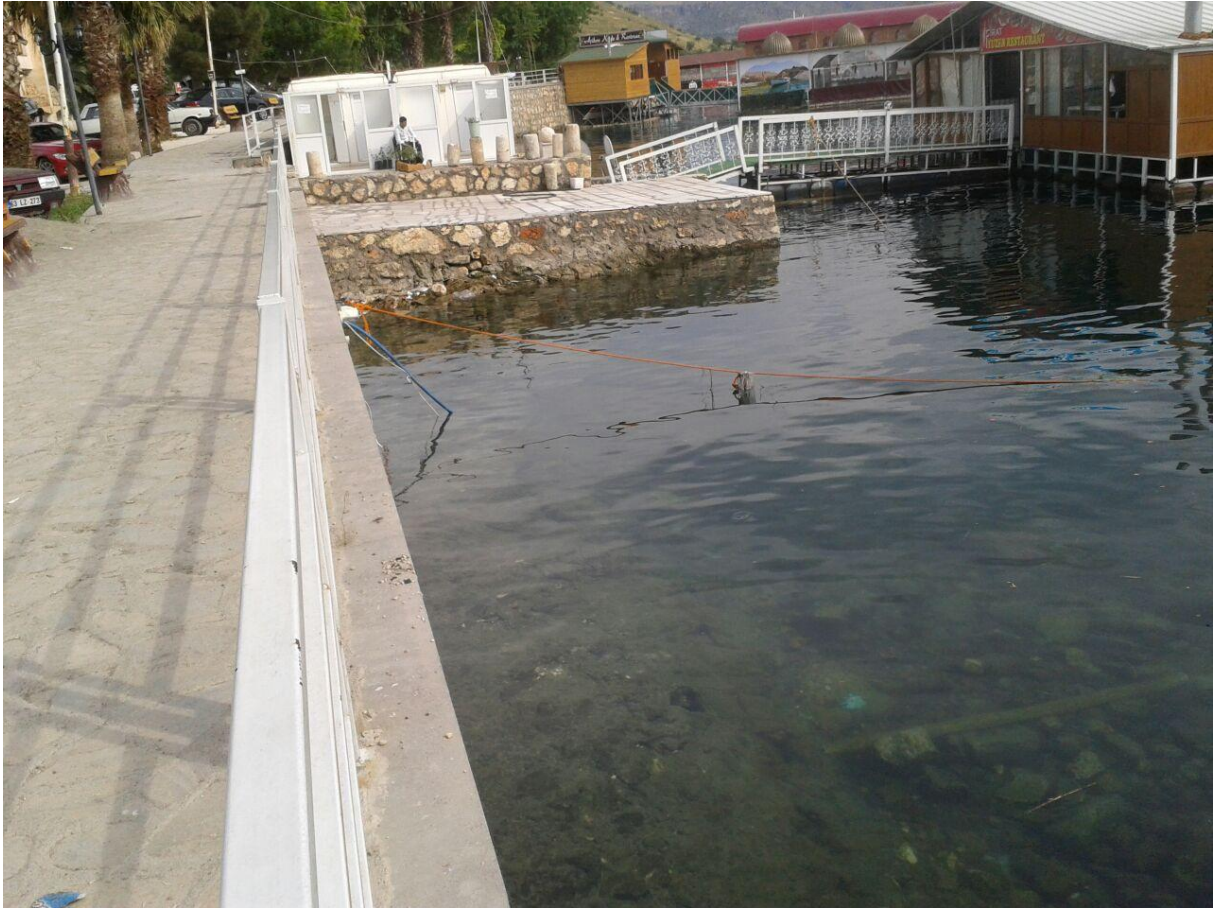
Photo 10. The Sewage of the restaurants (white shed in the photo is toilet of a restaurant) leaking to the river (Gülbandılar, 2015)
