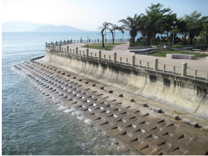
Figure 17. Concrete constructions around the northern section of Yersin Park at the river mouth of Cai river.
