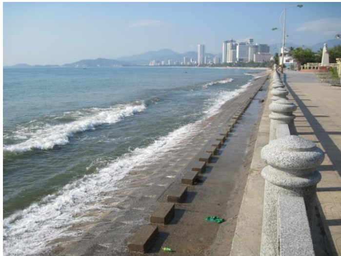
Figure 18. The groins are visible on the east stretch of Yersin Park. The picture is taken towards the south of Nha Trang.
