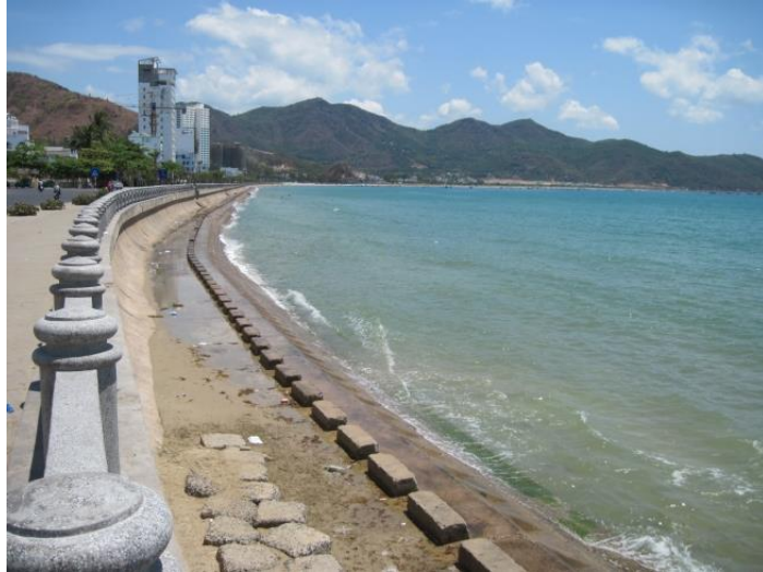
Figure 11. The beach of Cai river mouth has suffered from severe erosion and today the beach is absent and only the seawall is visible
