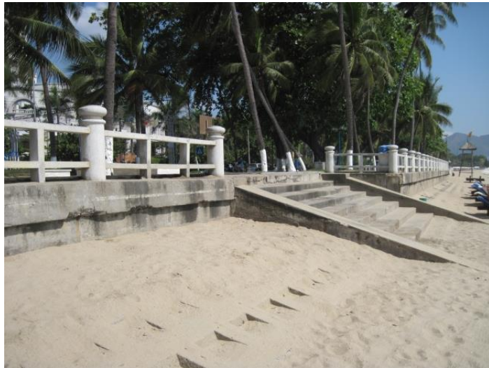
Figure 21. A part of the vertical and sloping seawall along the stretch between Nha Trang View restaurant and the structure Hoa Bien.
