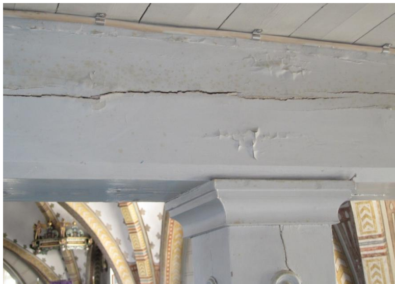
Figur 21 Sprickor i takbalk
