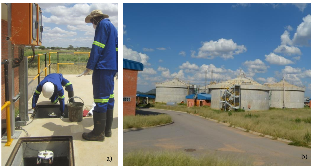
Figure 10.1. a) Sampling of primary sludge from buffer tank after anaerobic digestion, b) Anaerobic digestion tanks
