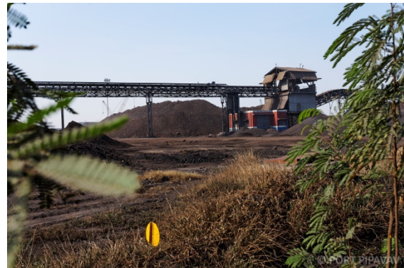
Picture 5 Conveyor belt to coal yard
