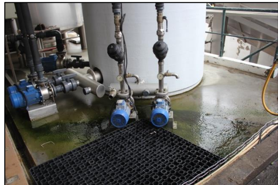
Picture 4: Example of leakages.
