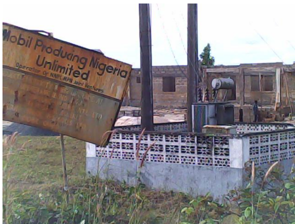
Electricity project at Ibenu
