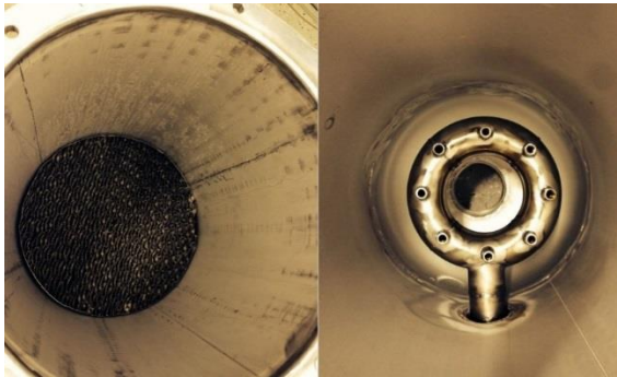
Figure 4.5 Packings and nozzles inside the humidification tower
