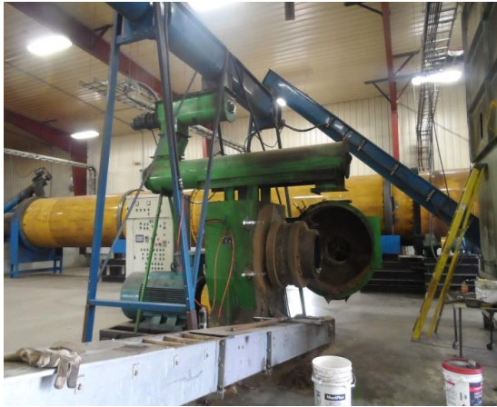
Figure 5-1: Equipment used to produce pellets at the Greenwald Hutterite Colony
