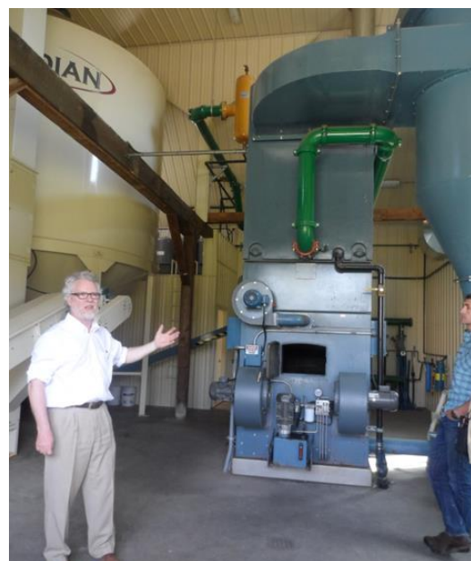
Figure 5-2: Blueflame stoker biomass burner installed at Providence biomass burner at Providence College
