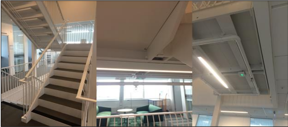
Figure 3.4. Staircase with absorbents under each tread.
