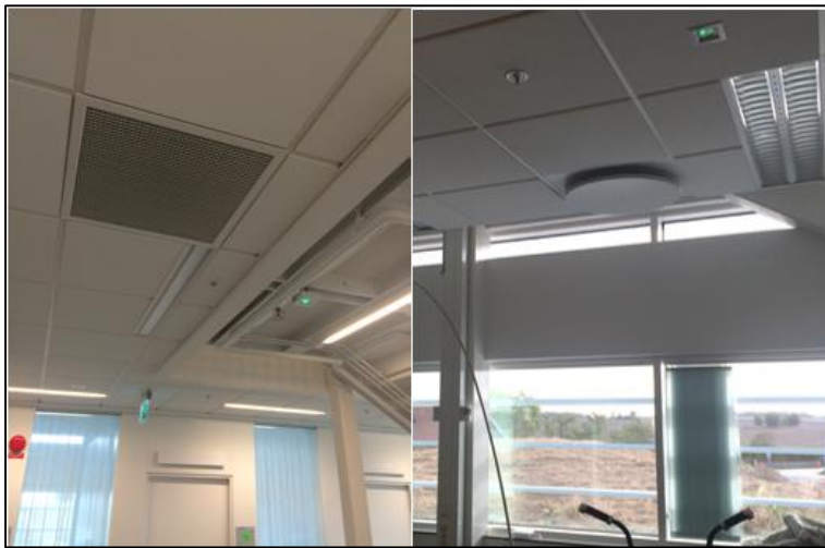
Figure 6.1. Possible installation causing background noise.
