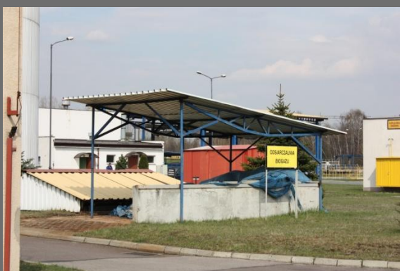
CLEANING FACILITY FOR RAW BIOGAS
