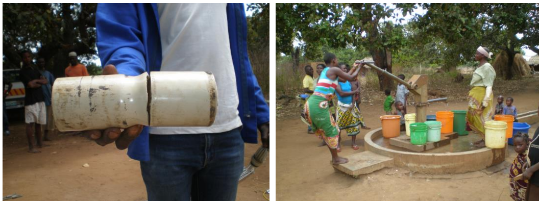
Figure 4-23 The crack in the pipe that made the pump non-functioning for a year prior to testing (left) and the now used pump (right).
