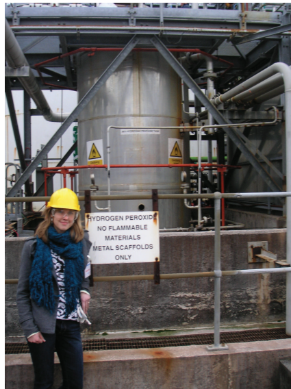
Figure 5.6: The tank to be controlled in Warrington.
