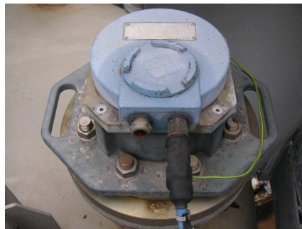
Figure 5.7: The radar level sensor of the tank in Warrington.
