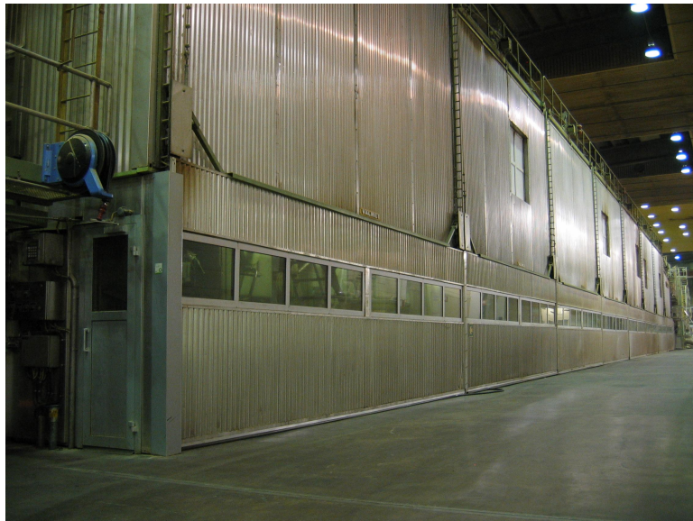
Figure 3.4: Dryer section hood at PM3. Photo by Choy-Hsien Lin.
