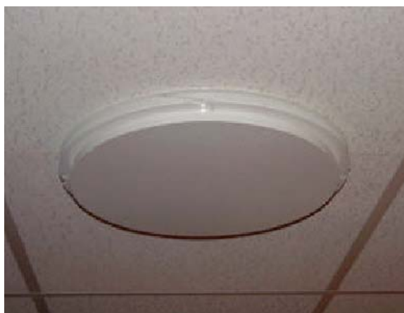
Figur 4.2 – IDCC monterad i undertak [F3]
