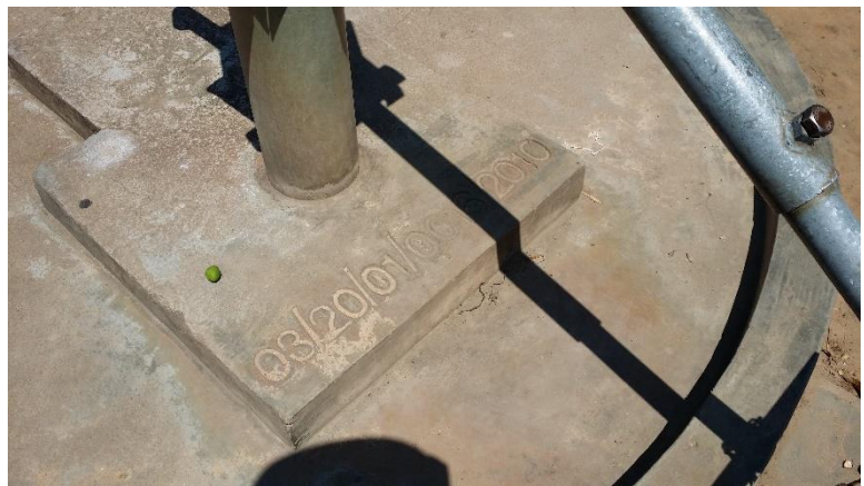
Figure 14 Borehole identification number stamped into the concrete foundation of the well. The well is called Cuhari B. Foto: Elin Olsson.
