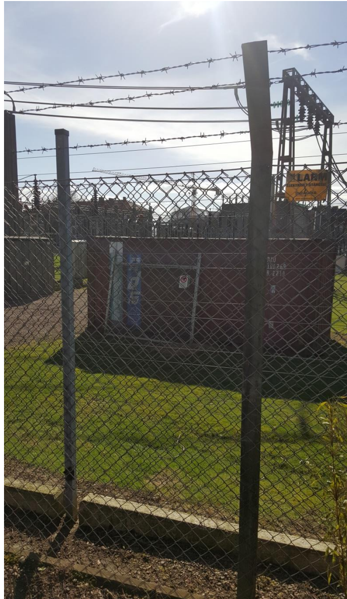
Figure 4. Example of the fencing around substations.
