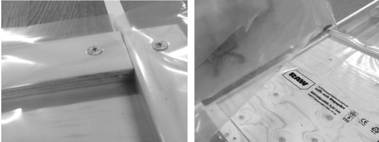
Figure 9 - From left to right: plastic sealed corner of the form and the completed form with a plastic cover attached to it.
