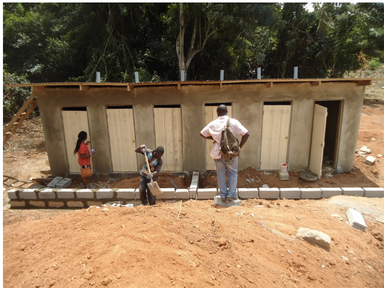
Figure 6 Example of a KVIP. PVC piping vents the latrine pit to reduce smell and flies.
