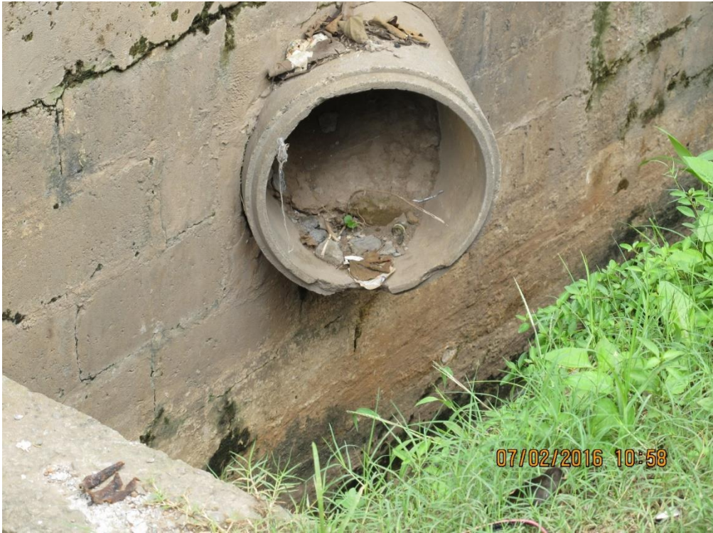
Figure 39: Image showing silt build-up inside the pipe due to lack of maintenance
