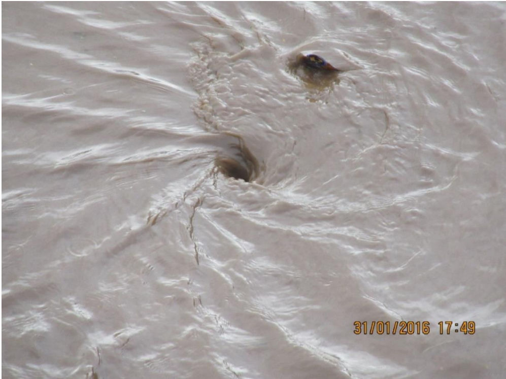
Figure 42: Two gullies when there was flooding (31/01/16) about an hour after Figure 41 image was taken
