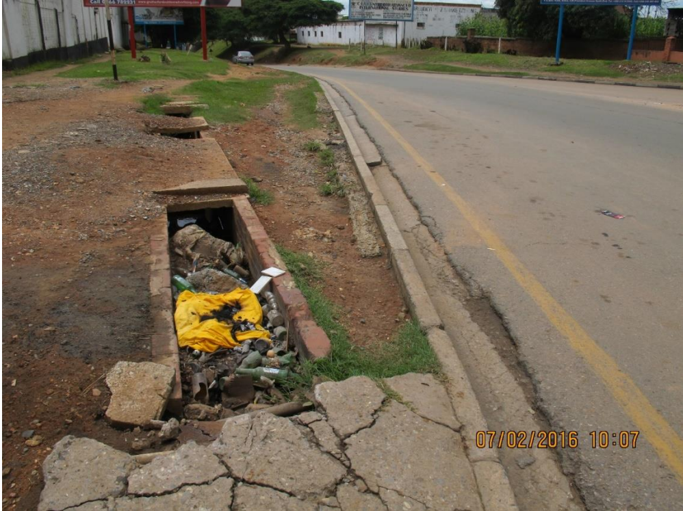
Figure 26: Fully blocked drainage at the junction of Maina Soko road and president avenue
