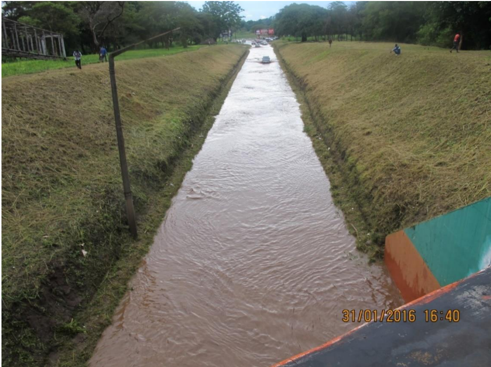
Figure 41: Flooding but two gullies cannot be seen due to depth of water (surcharge)
