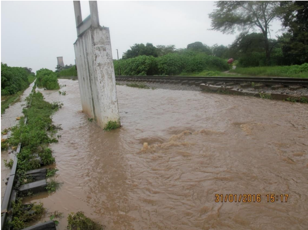
Figure 23: Flooding along the rail right above the underbridge in eastern direction
