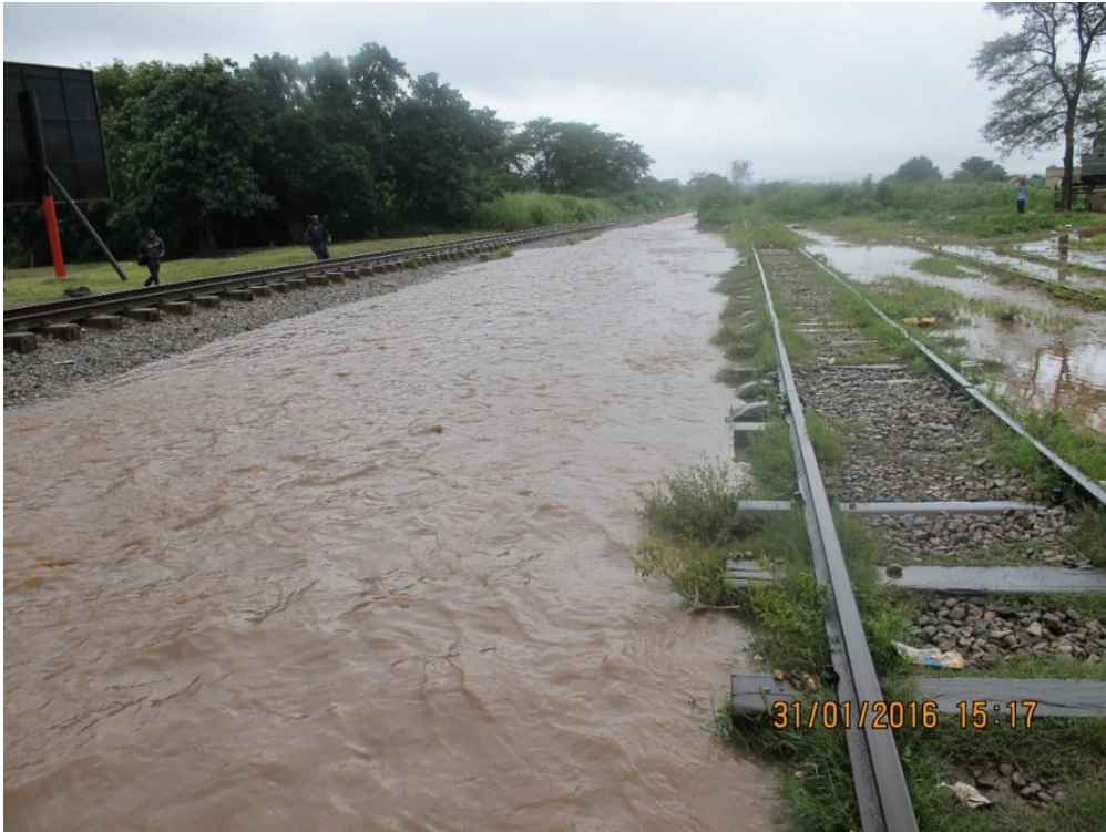
Figure 22: Flooding along the rail right above the underbridge in western direction
