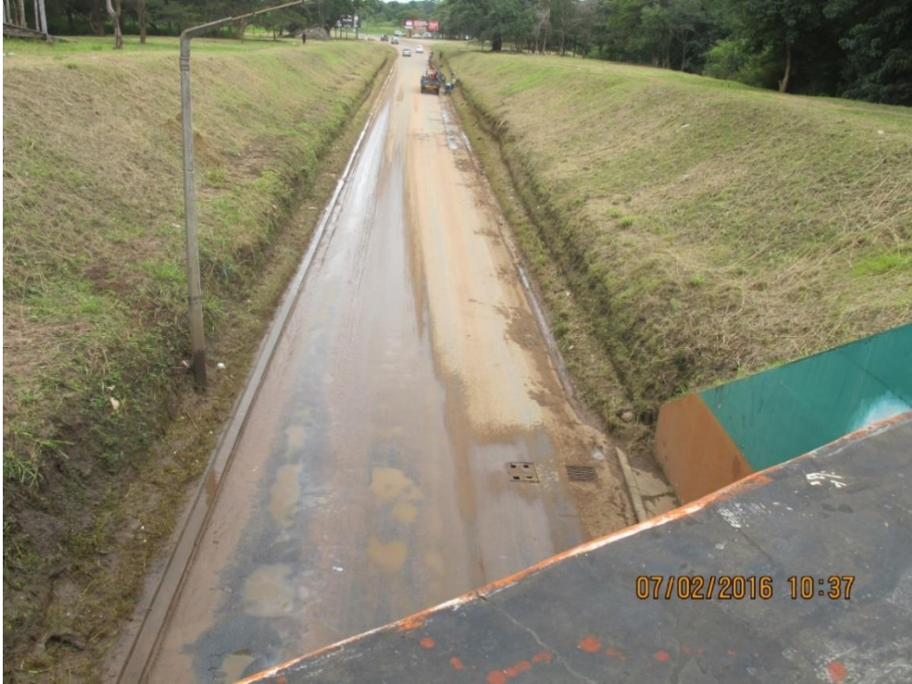
Figure 40: Earthen embankments with two gullies when there is no flooding
