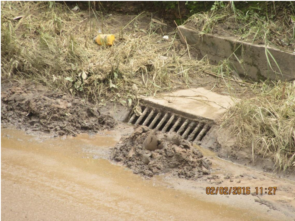
Figure 38: Silt build-up 2 days after the flood (31/01/16) causing blockage to the gulley and eventually pipes as shown in Figure 39 if not maintained
