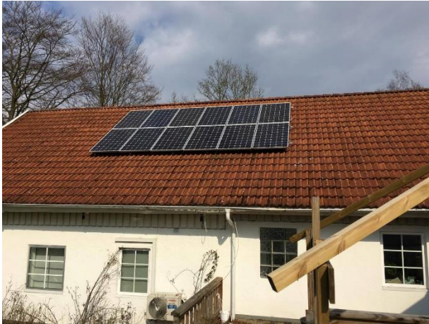
Figure 13. Picture of solar panels of one of the customers.
