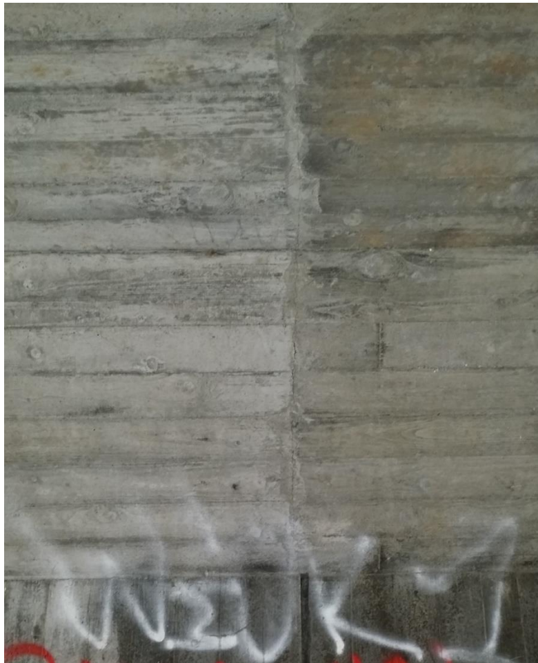
Figure 99 – Crack in bridge 12-1374-1. Only a single crack in the construction join for the valve was found.
