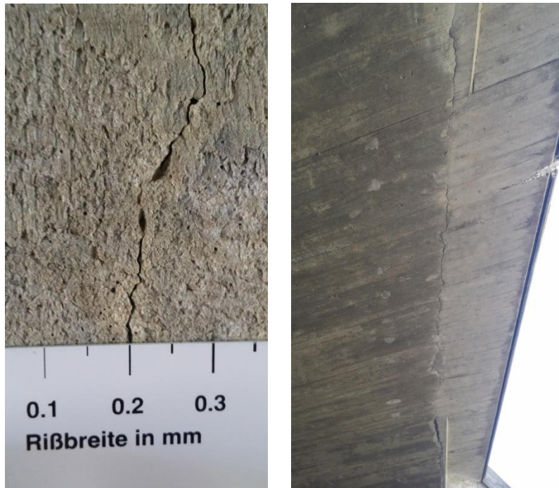
Figure 90 - Cracks in bridge 12-404-1. Left is front wall and right is valve.
