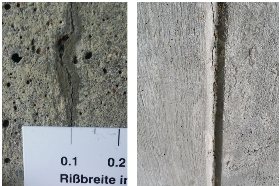
Figure 91 - Cracks in bridge 12-438-1. Left is front wall and right is construction join for front wall.
