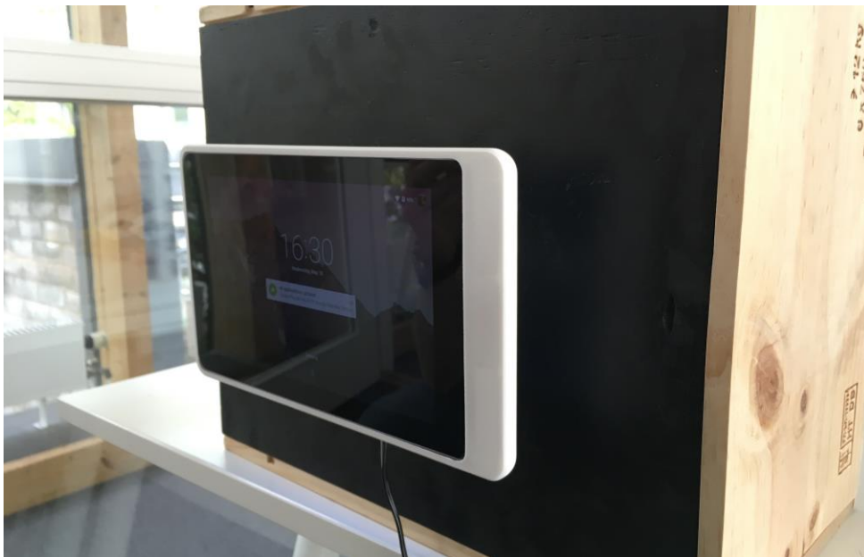
Figure 11.2 The CP docked and charging on the demonstration box.
