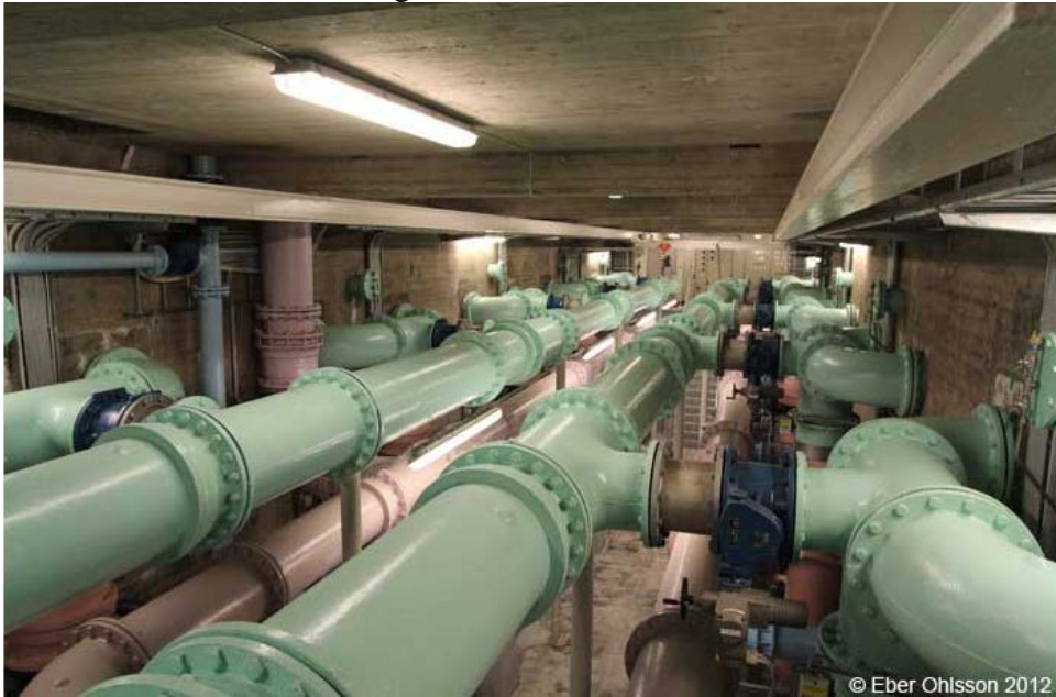
The interior of filter building 2
