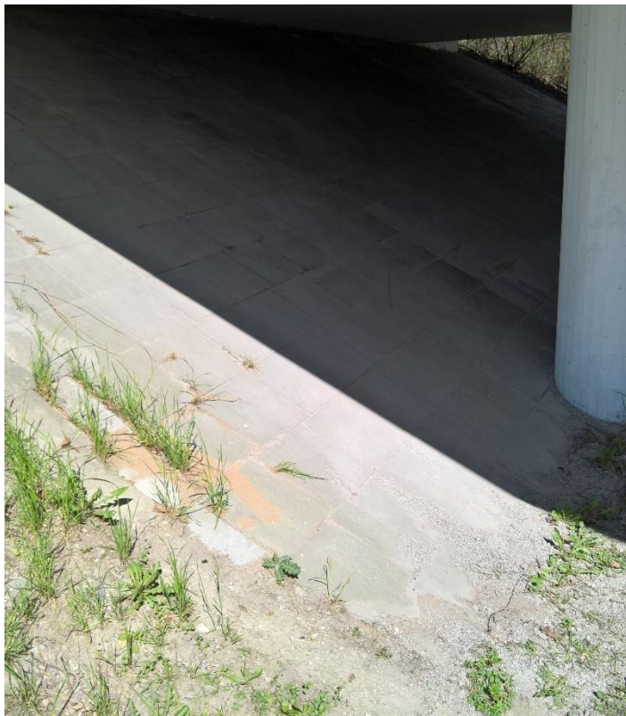
Figure 48 dusty concrete test
