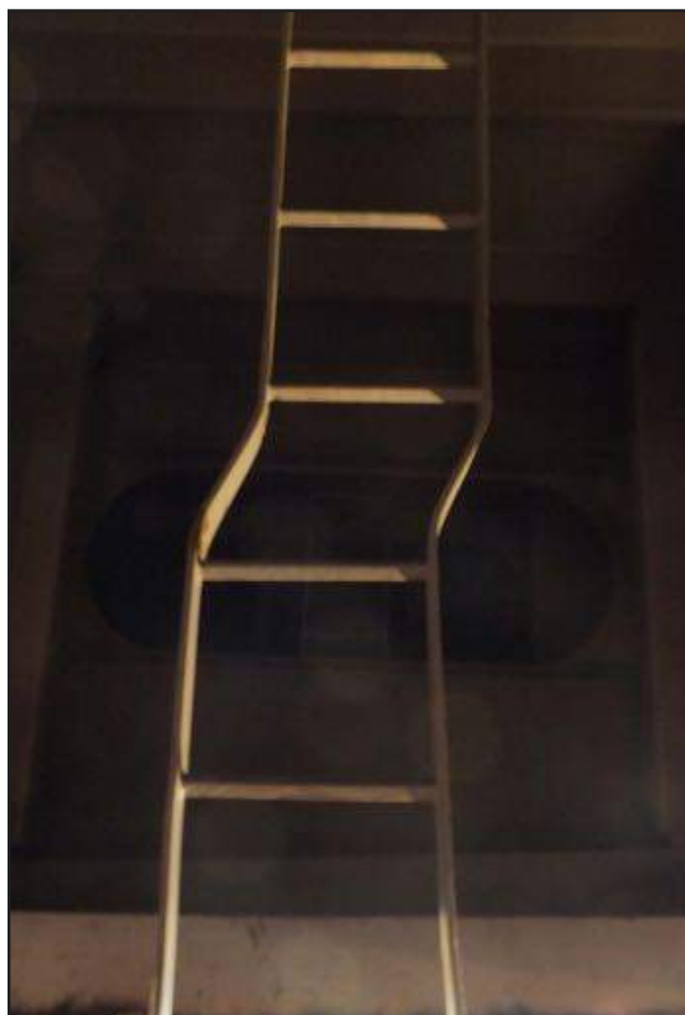
Figure 12: Example of internal ladder damage in a void space
