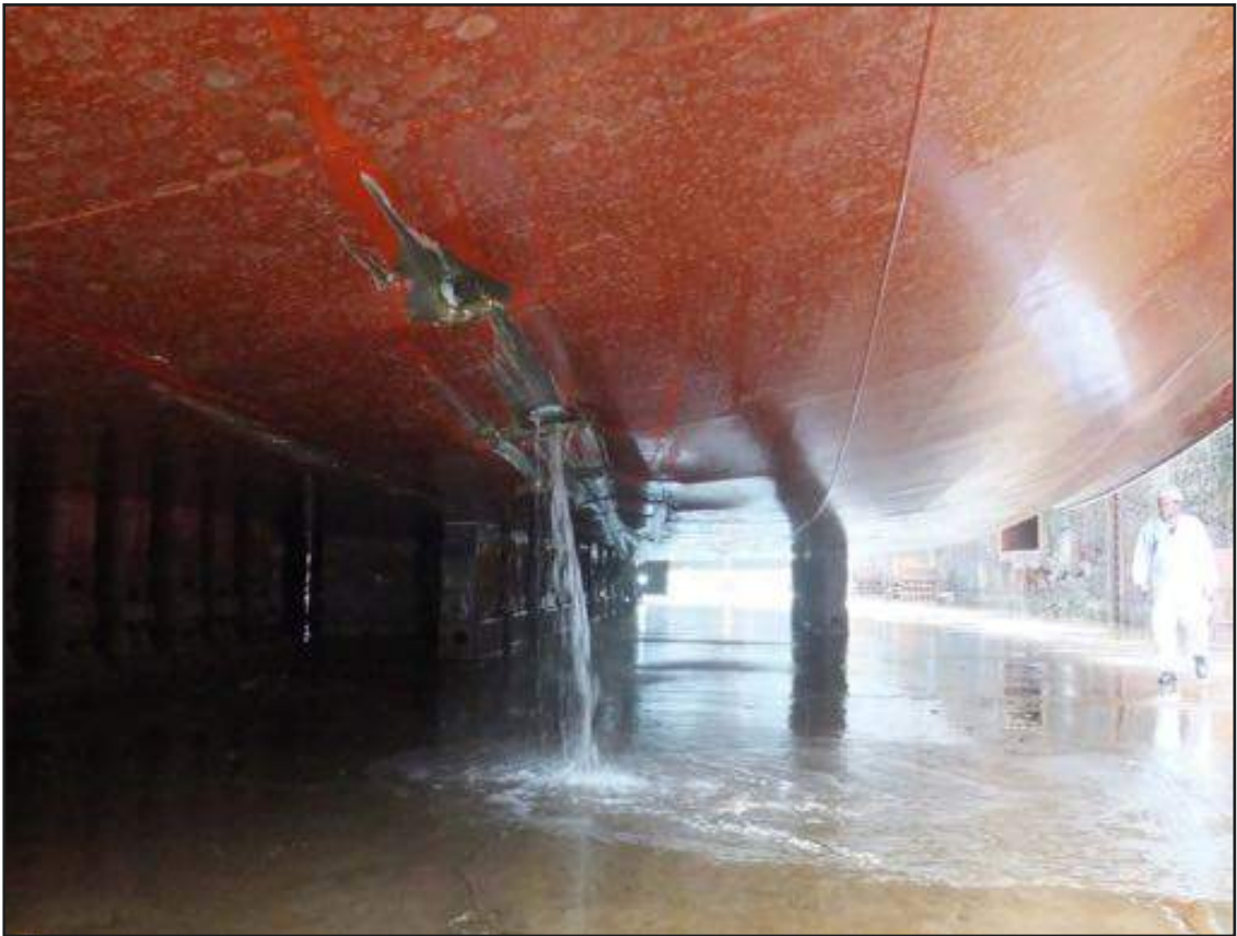
Figure 7: Hull gouging looking aft
