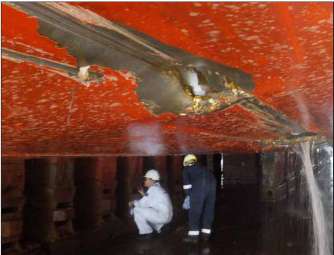
Figure 8: First hole in water ballast tank 4
