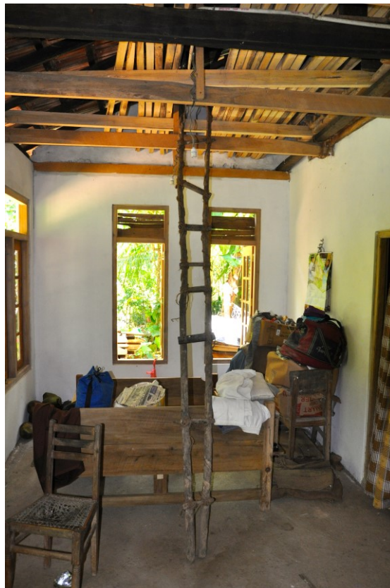
Figure B 2 – A ladder which was used by a family to reach the suspended ceiling when the house was flooded.
