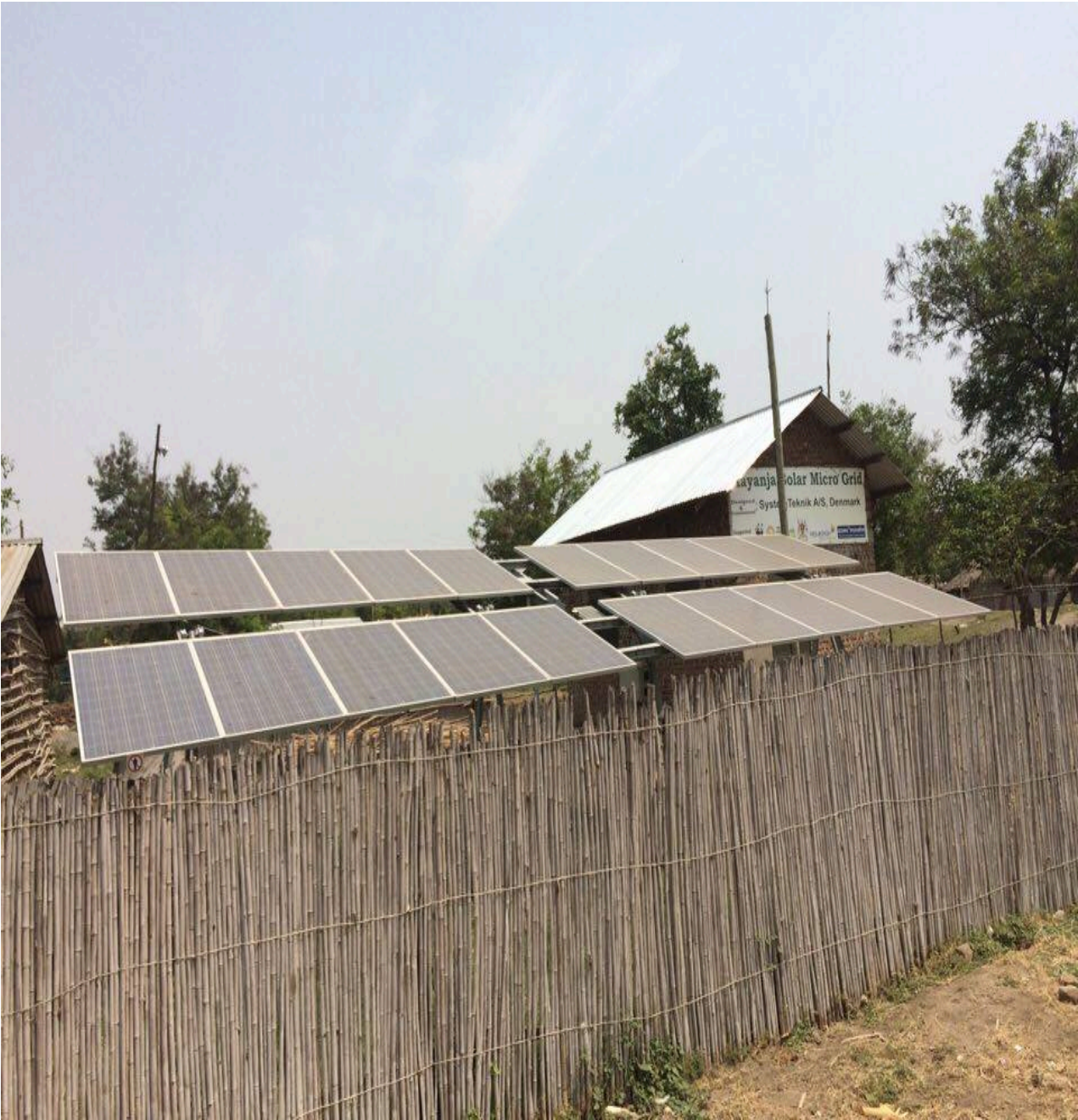
Appendix C: Systems teknik (Denmark) powered Kayanja Solar Mini-grid power installation seen from a distance. All photos by researcher.
