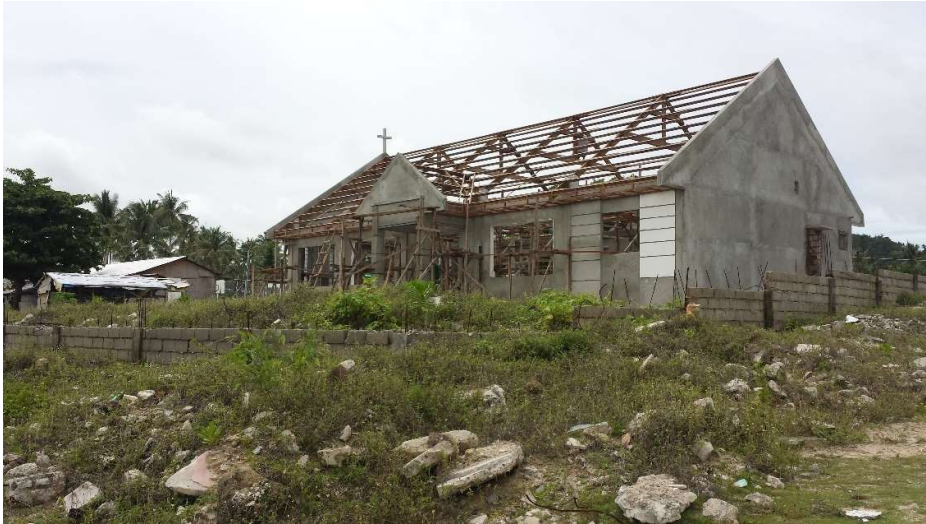
Figure 12. The new church under construction just a few meters away from the previous one.
