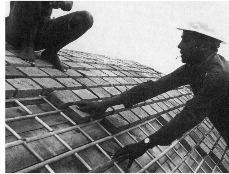
Figure 40: Photograph of Builders composing a curved roof of an Eladio Dieste project
