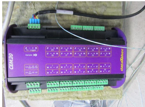
Figure 25: Data logger expansion - CEM20 dataTaker
