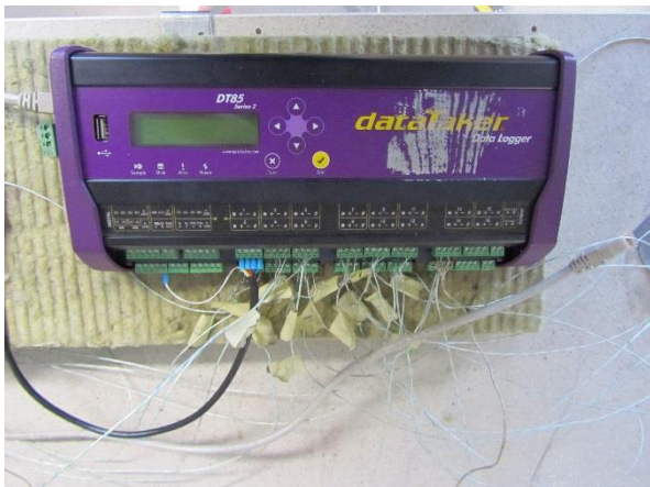
Figure 24: Data logger - DT85 dataTaker
