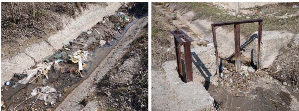
Figure 9. Showing a highly littered and sedimented channel immediately downstream of the enclave (left) and broken channel gates (right) in Khalmion WUA (03/17).
