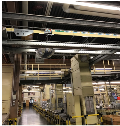
Figure 19. Overhead ceiling conveyor system
