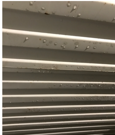
Figure 30. Container rain observed on container’s ceiling
