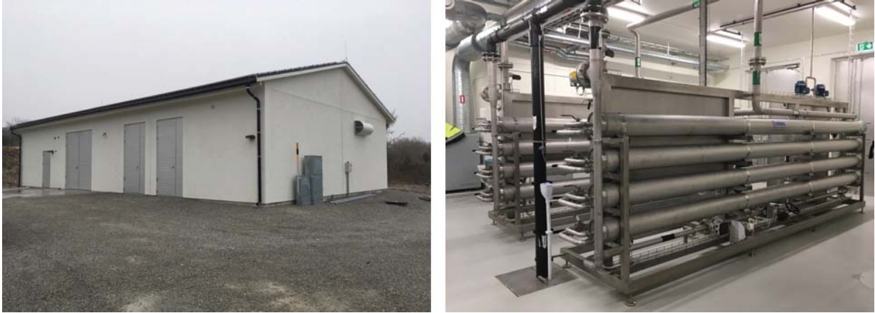
Figure 4. Desalination plant in Herrvik from the outside (left) and the membrane filter inside (right). Own photographs.
